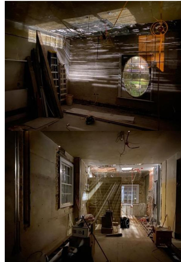
IMAGES OF THE UPPER FLOOR OF THE OLD LIBRARY DURING CONSTRUCTION WORKS.
